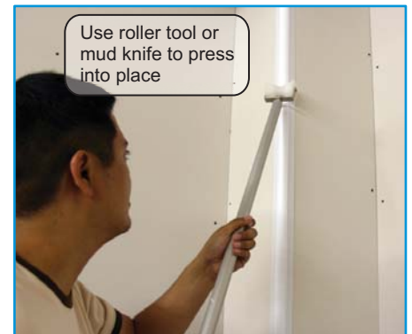
Place bead onto drywall corner once mud is troweled or boxed on
